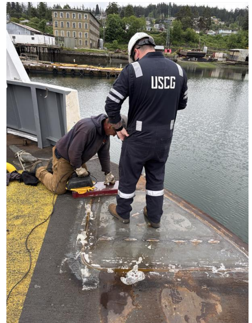
U.S. Coast Guard witnessing vacuum box testing of the welds on the steel inserts on the car deck
